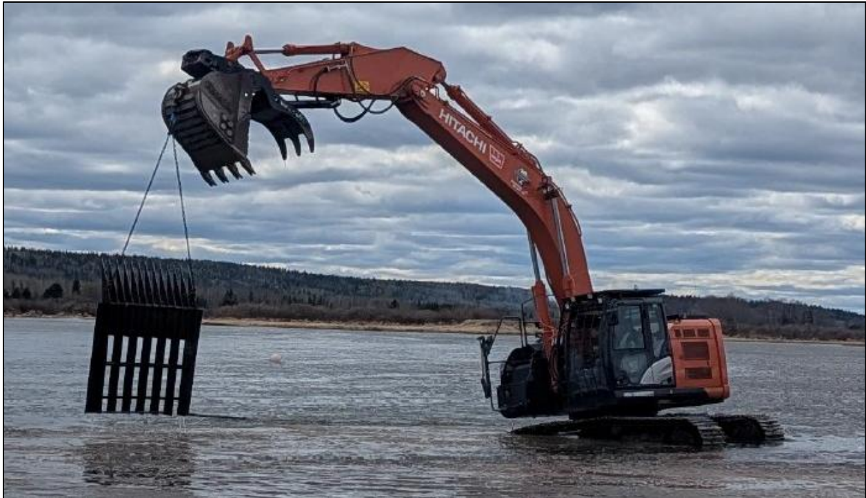
Photo 1.2 Sled used during the larger-scale restoration of the Lower Patch on May 5-10, 2025; a boom extension was also used for greater reach (not shown).
