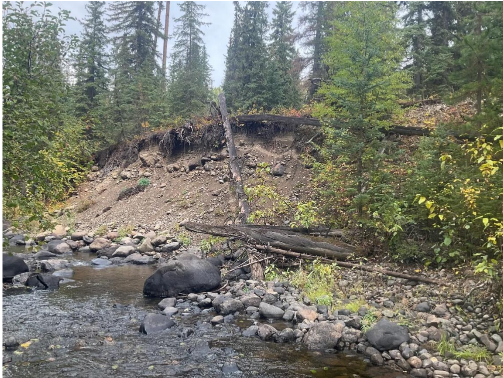
Appendix Photo D-29. Steep, eroding bank contributing sediment load at SW3. September 24, 2025.
