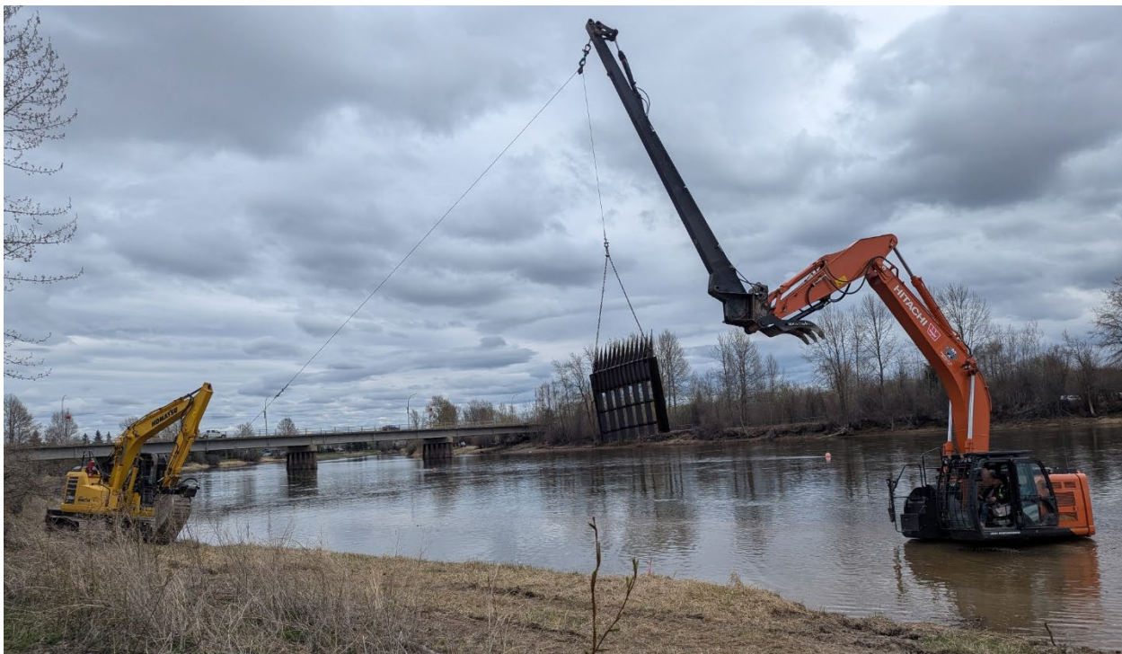
Figure 7. Testing operation of the sled using a winch and pulley system, May 2025.
