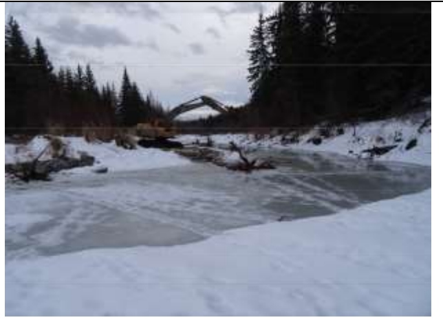
Photo 42. Root wads and boulder clusters being installed on the North bank looking upstream to the North.
