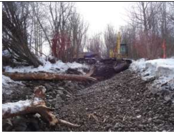
Photo 15. Sloping channel bed to simulate natural stream morphology. Note the dump truck in the background transporting soil removed from the historic channel.
