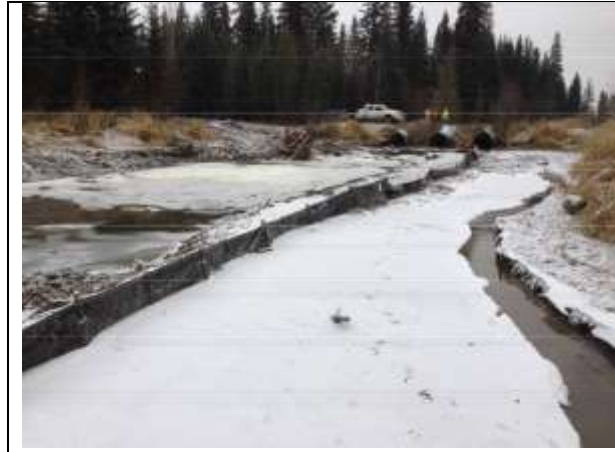
Photo 14. Isolation of area to be dredged and enhanced with fish habitat structures. Note the diversion channel to the right of the photo.
