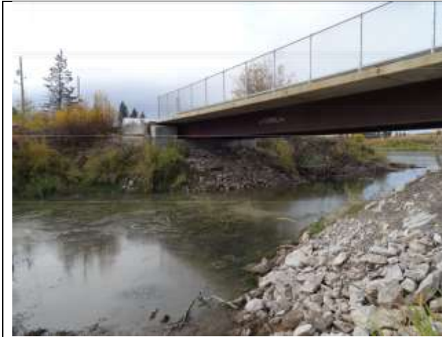
Photo 29. Stoney Creek at the Douglas Street bridge/Nechako River confluence illustrating the bank erosion occurring upstream of the bridge.
