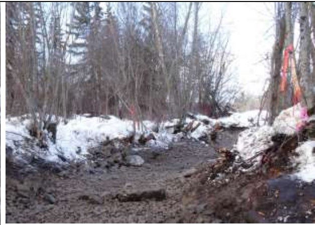
Photo 14. Alder tree stumps and roots left to provide bank stability, create undercut bank refugia and sprout new shoots.
