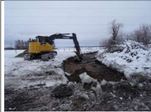
Photo 9. The excavator operating from a protective layer of snow and ice atop frozen ground downstream of the alder grove.
