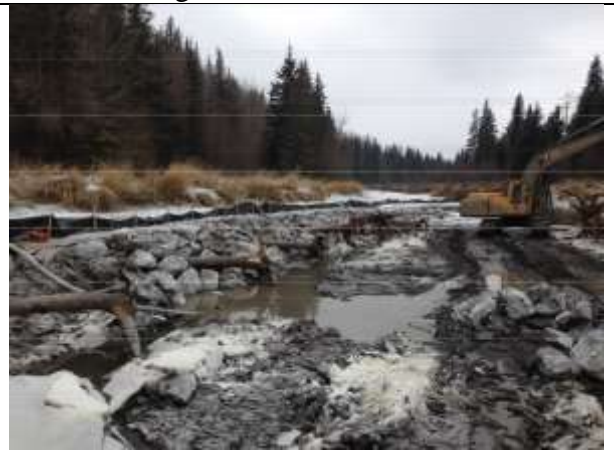
Photo 17. Armouring of the channel. All root wads were anchored to boulders with 1/4 inch cable.
