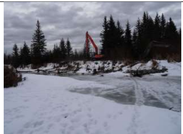
Photo 44. Boulder Clusters and root wads being placed from atop of the North bank.
