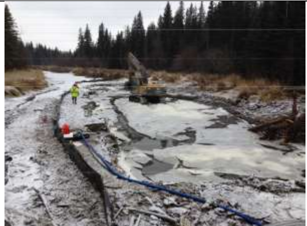
Photo 15. Beginning of dredging along the North bank with area fully isolated with flow diverted along the South bank
