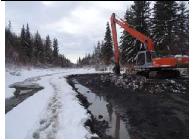
Photo 48. Area immediately upstream of the beaver dam being dredged. Note the earthen platform from which the excavator is being operated and away from the wetted channel.
