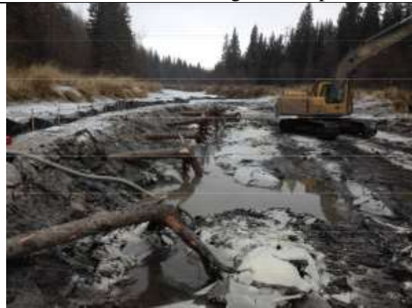
Photo 16. Installation of root wads (LWD) that will provide cover, create scour to maintain pool depth, and capture debris.
