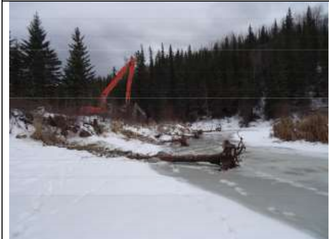
Photo 41. Root wads and boulder clusters being installed on the North bank looking upstream to the West.
