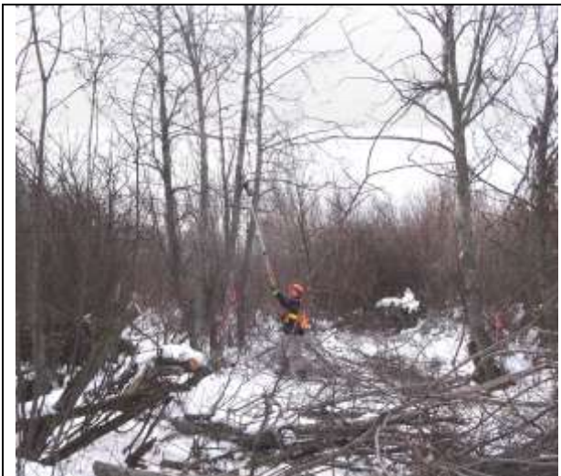
Photo 11. Alder branches overhanging the historic channel carefully being removed to create a path for the excavator.
