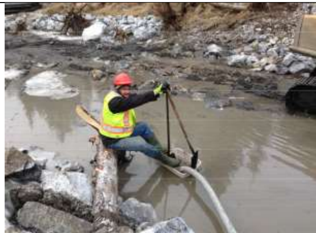
Photo 19. Pumping of turbid water into the riparian habitat with a fish-friendly intake.
