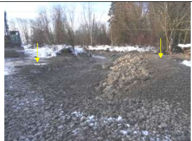
Photo 24. Top of the north bank and transportation route seeded with Vanderhoof Roadside Mix ® looking downstream.
